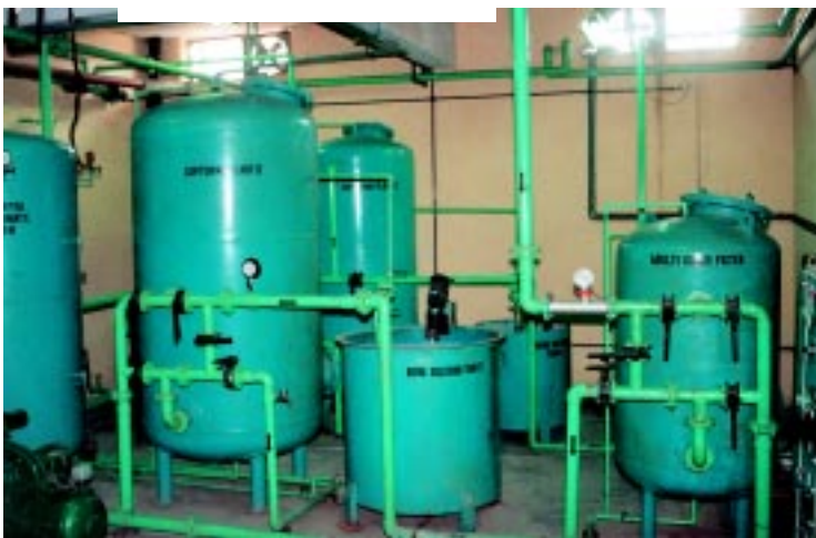
Times of India, Ghaziabad – multigrade filter, dosing system and reverse osmosis plant.
