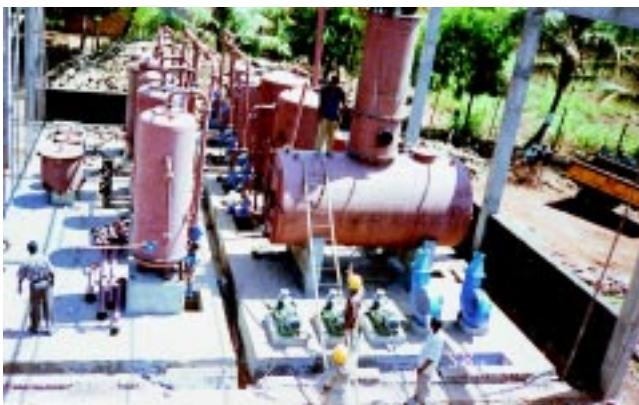
Water treatment plant for 20 MW cogen unit of Shree Doodhganga Krishna Sahakari Sakhar Karkhane Niyamit, Dist. Belgaum, Karnataka.
