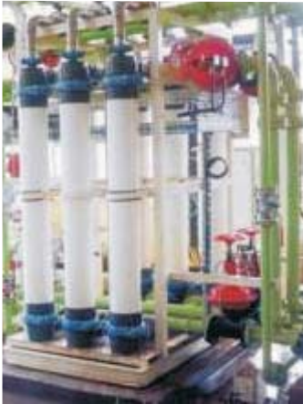
Ultra filtration plant
