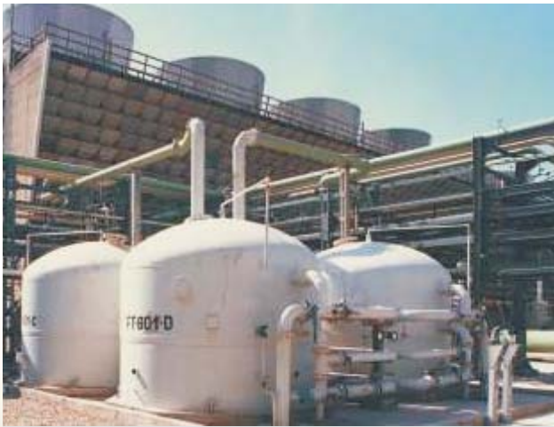
Cooling water treatment
