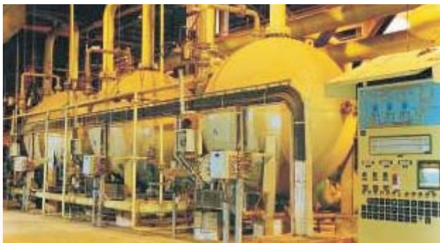
Condensate polishing units
