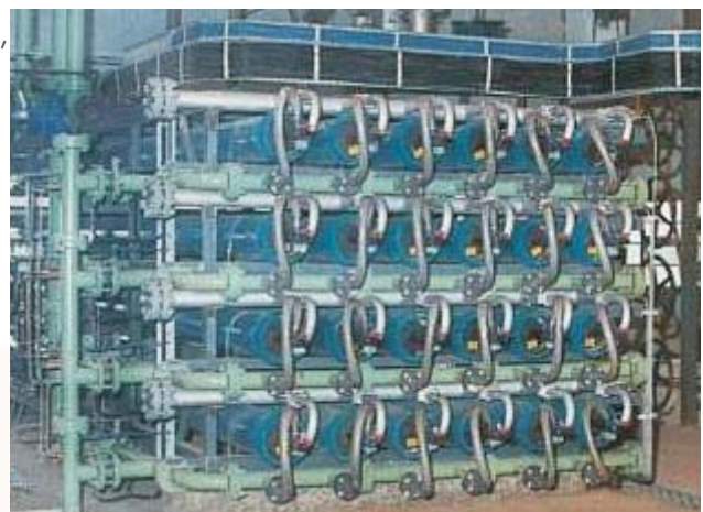
Sea water reverse osmosis desalination plant
