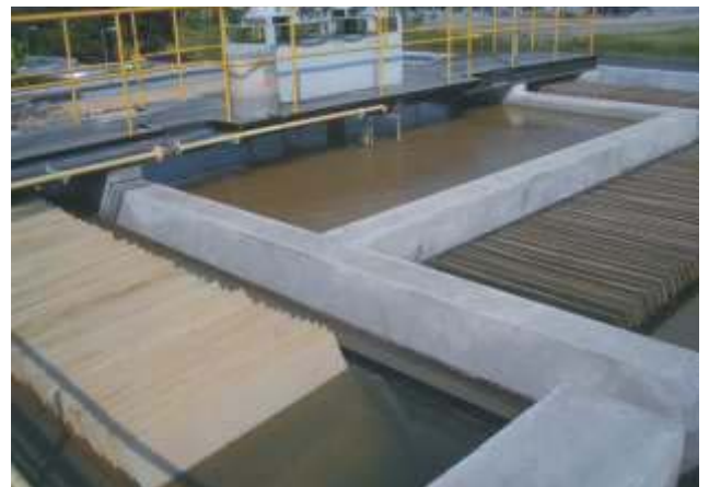
Ultra high rate clarifier
