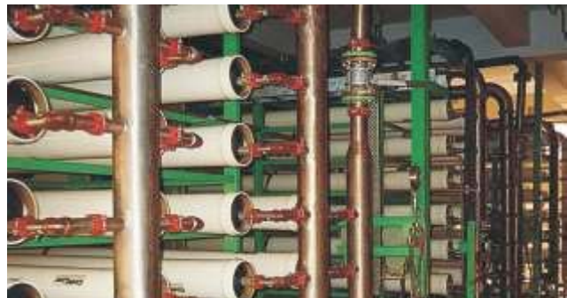
Zero discharge plant
