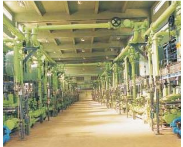
O & M services at power station
