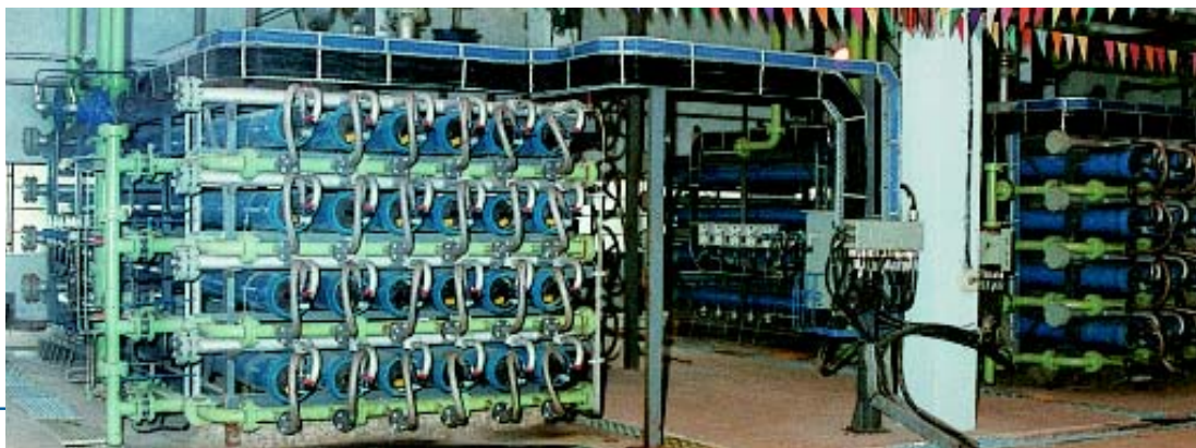
Sea water reverse osmosis desalination plant.
