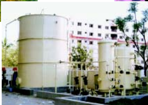
Fluidised media reactor for sewage treatment
