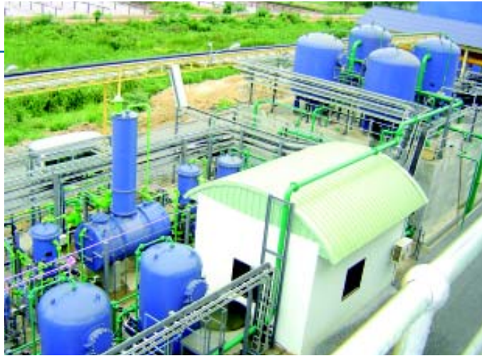
Water treatment plant (softening, demineralisation, condensate polishing and side stream filtration) for power project
