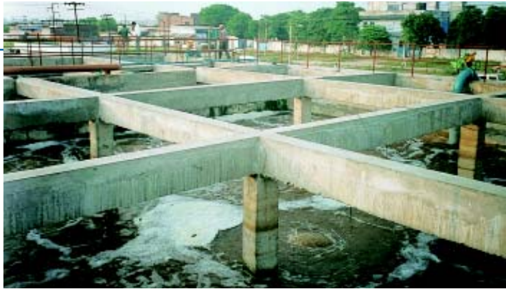
Sequential batch reactor for brewery effluent treatment
