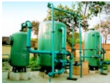
45 m 3 /h iron removal and softening system at Military Engineering Services' Dumayun Army Housing Complex, Garden Reach, Kolkata.
