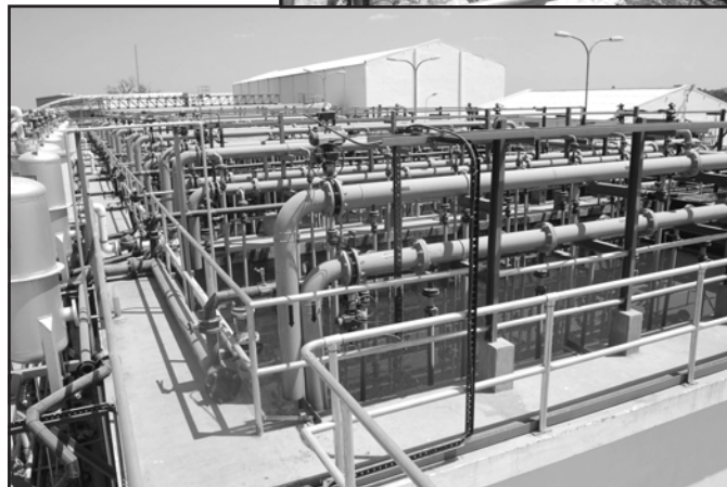
MBR section of 10 MLD zero discharge plant
