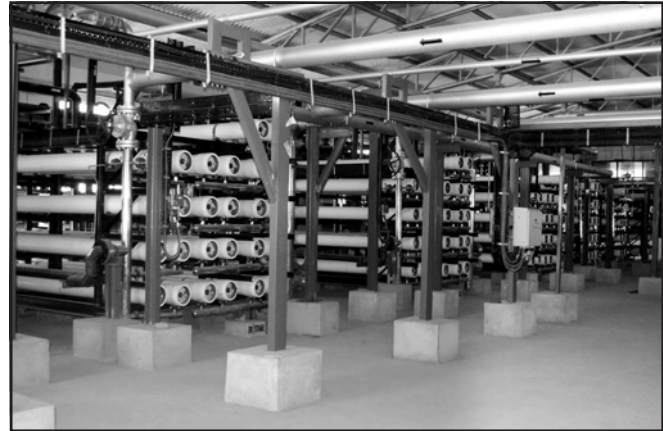
Reverse osmosis section
