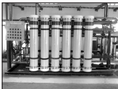
Ultra filtration section
